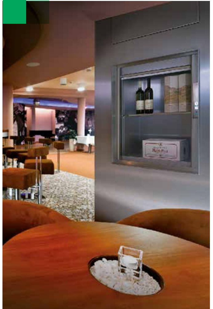
Installation in a bar (Spain), model 50 kg with stainless steel cladding.
